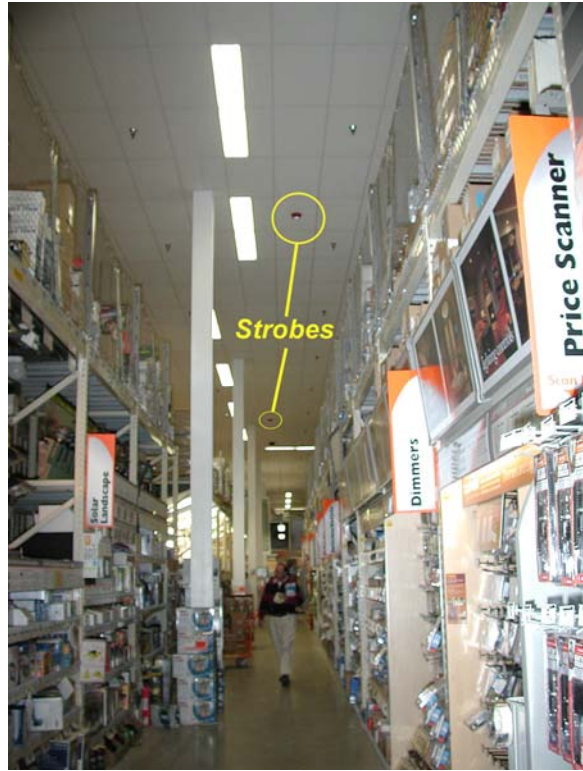
Photo 4 - Strobes Over Aisle
